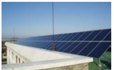
90KW Busan Water Pressure Control Center South Korea Roof Top Type
