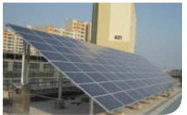
90KW Busan Metropolitan City Office of Education South Korea Roof Top Type
